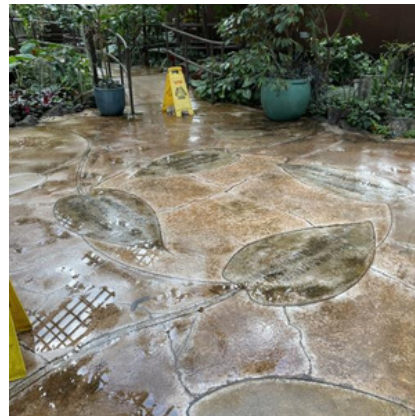
ID: Photo showing a wet floor with puddles of water and a yellow caution sign.
